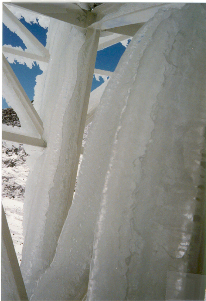
Figure 24. 12 cm of ice buildup in the reflector backup structure, 6 Jan 93.
