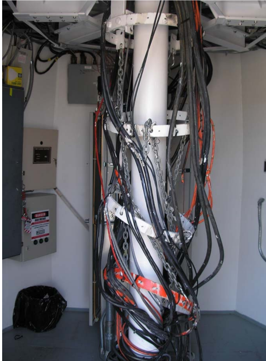
Figure 1. Maypole Cable Damage
