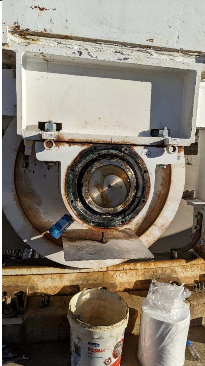
Figure 8: Azimuth Drive Axle Bearing Grease Inspection
