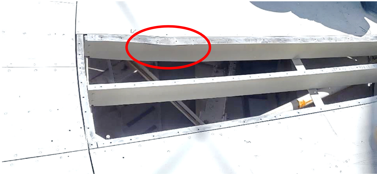
Figure 6: Doubler strip and Deformed Under-Structure
