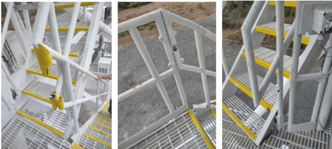
Figure 6: Hand Rail Corrosion Examples
