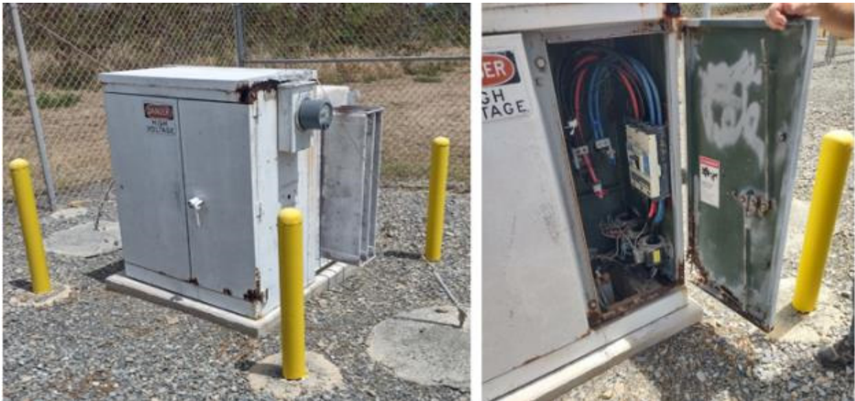
Figure 17: Site Transformer Condition
