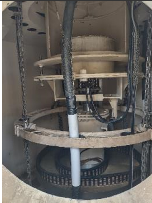
Figure 4: Upper Pintle – Cable Wrap Area Condition
