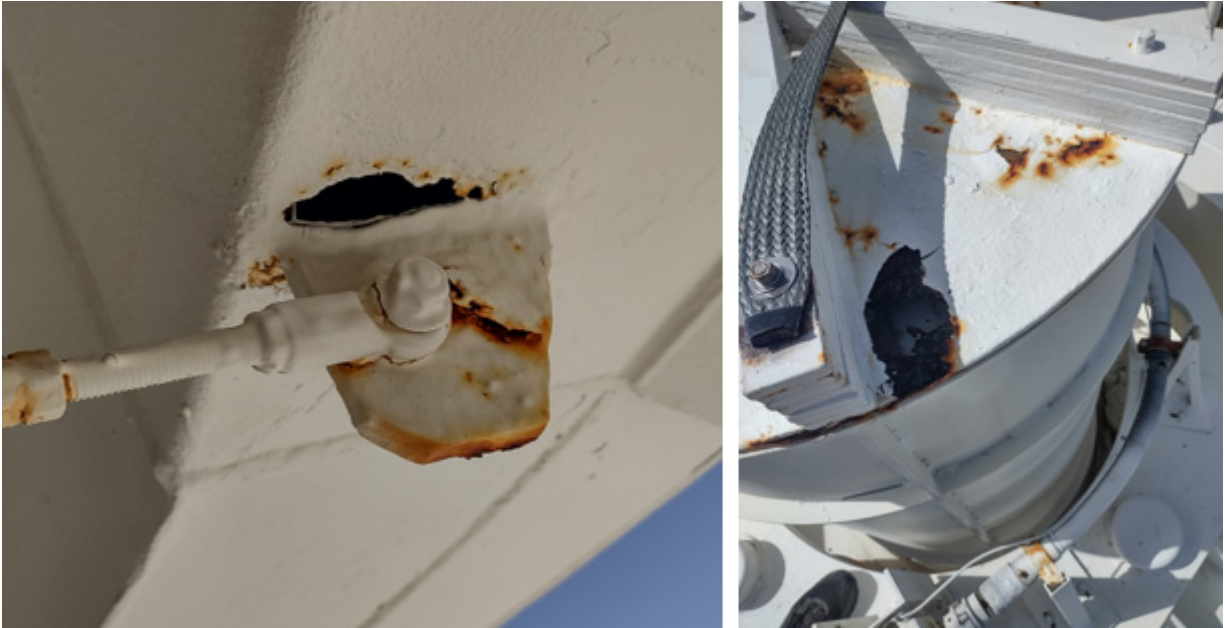
Figure 15: Apex Structure Rust Out
