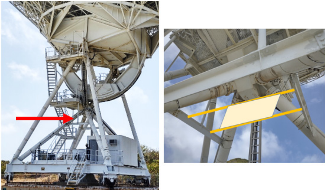
Figure 5: Lower Service Platform Needs Replaced
