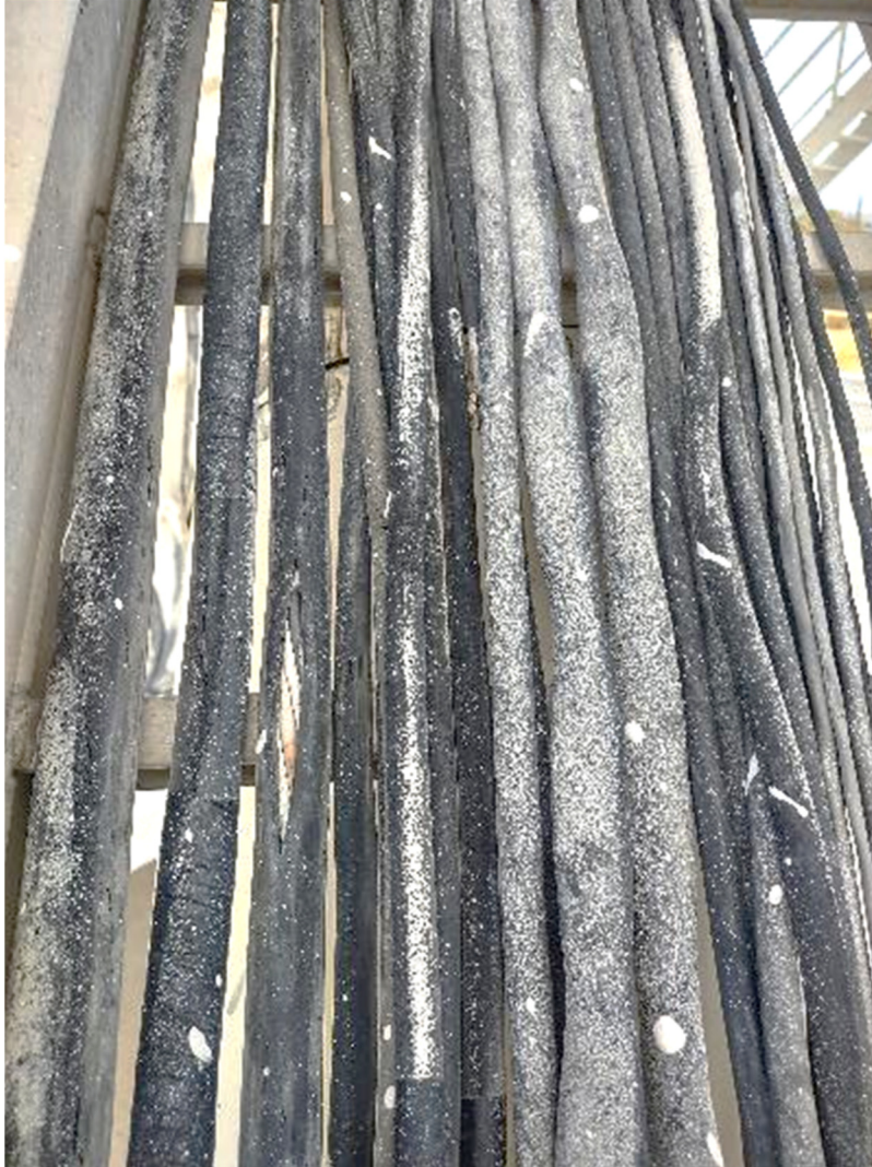
Figure 19: Antenna Wire Condition
