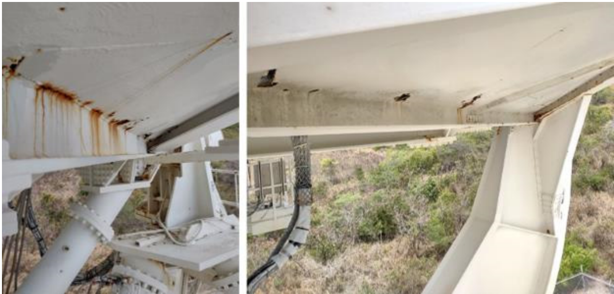
Figure 10: Box Areas that Need Repaired
