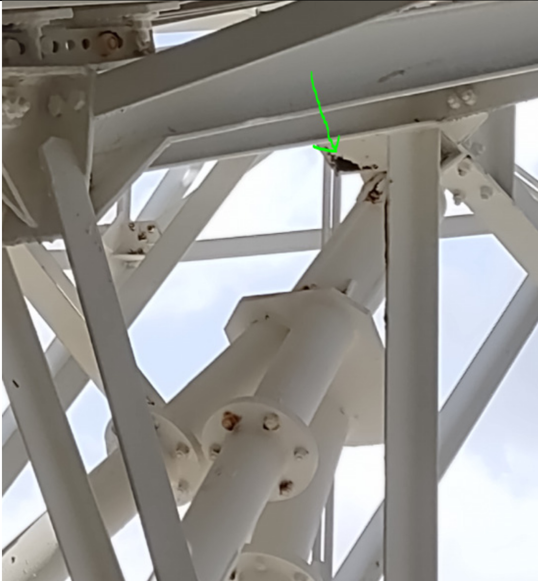
Figure 12: FRM Quad Leg Support Structure Rust Out
