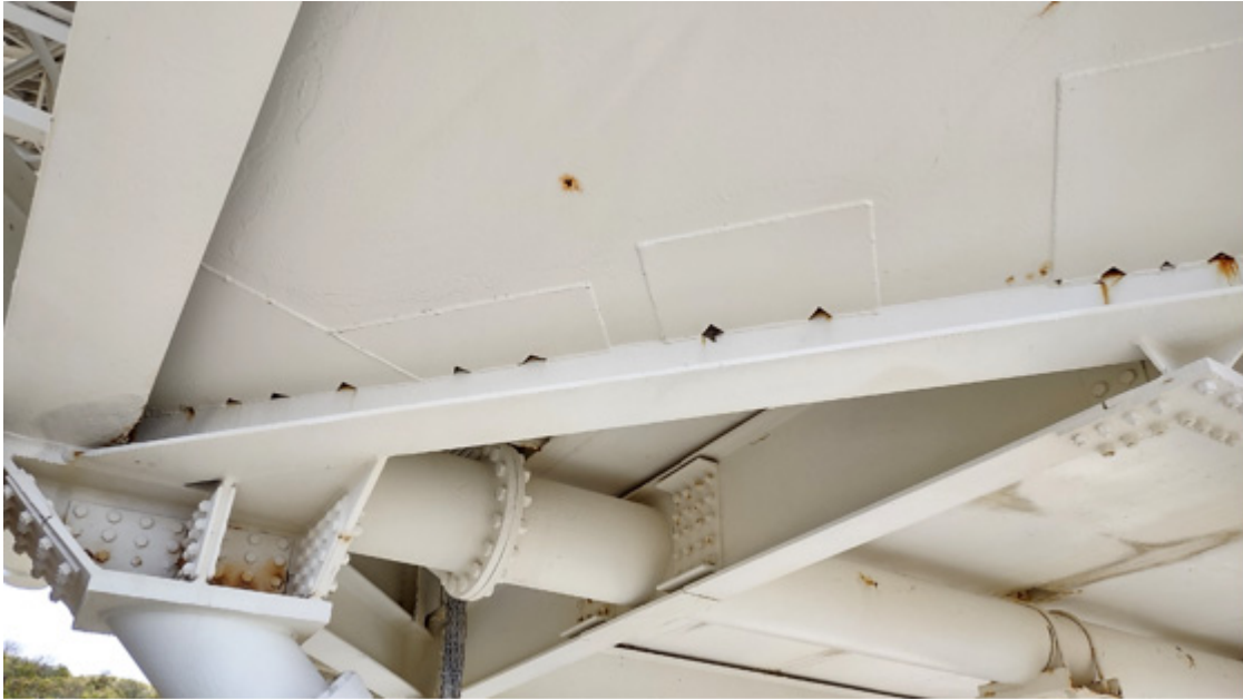
Figure 9: Condition of Past Repairs to one of the Box Areas
