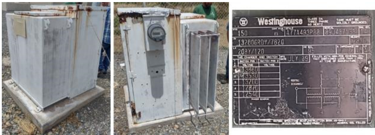
Figure 18: Site Transformer Condition
