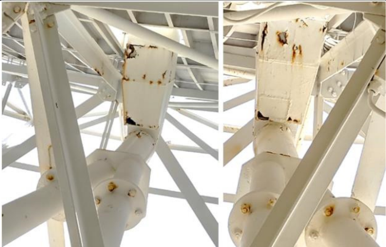
Figure 13: FRM Quad Leg Support Structure Rust Out
