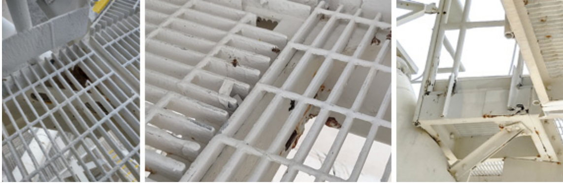
Figure 7: Walk Way Under Structure Corrosion Examples
