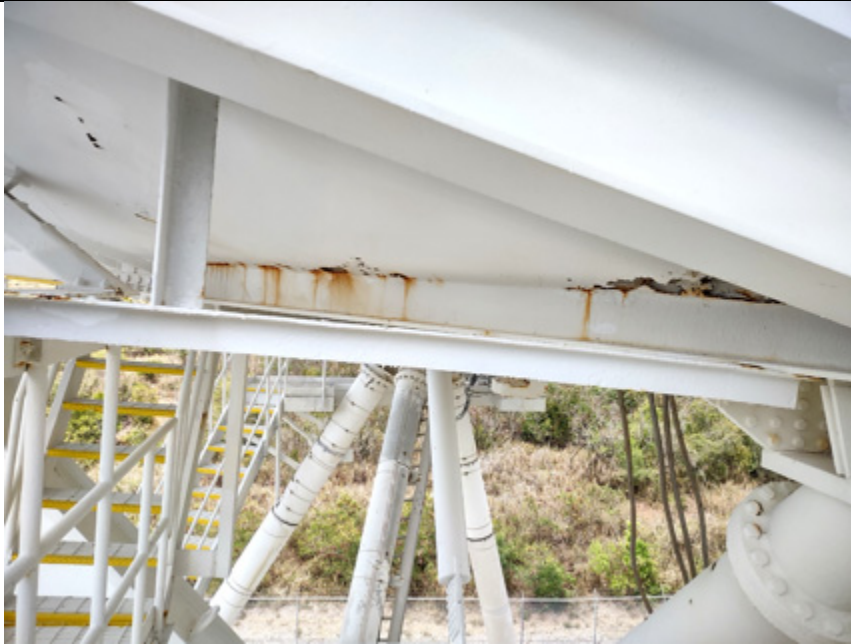
Figure 11: Box Areas that Need Repaired
