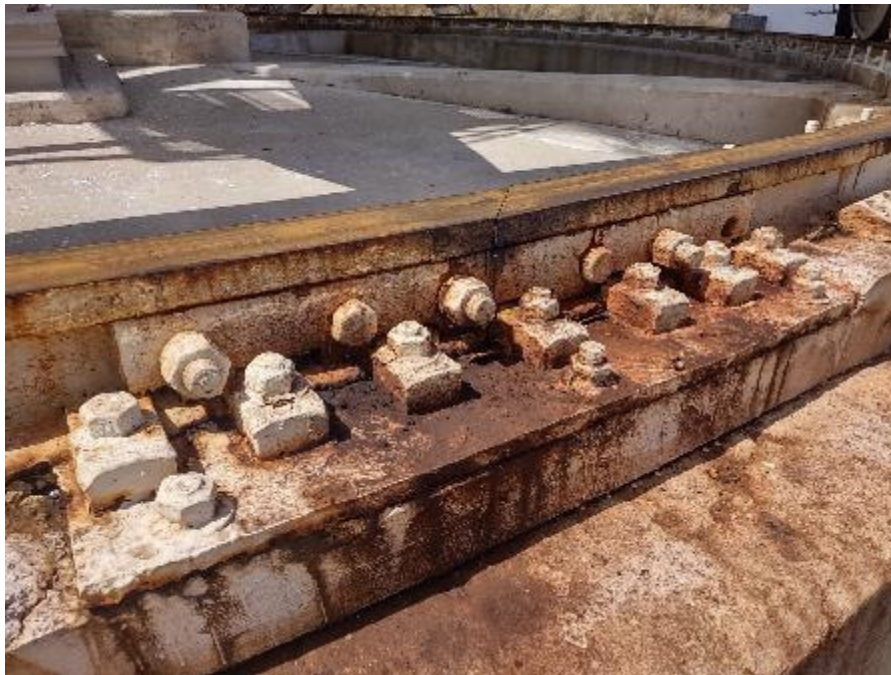
Figure 21: Splice with Significant Vertical Rail Movement
