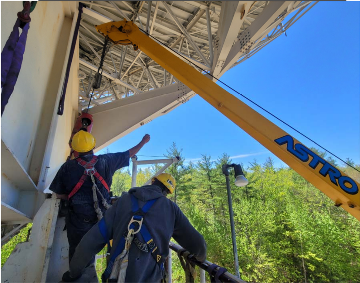
Figure 7: Mechanics work with the crane operator to hoist the pillow block up and out of the antenna.
