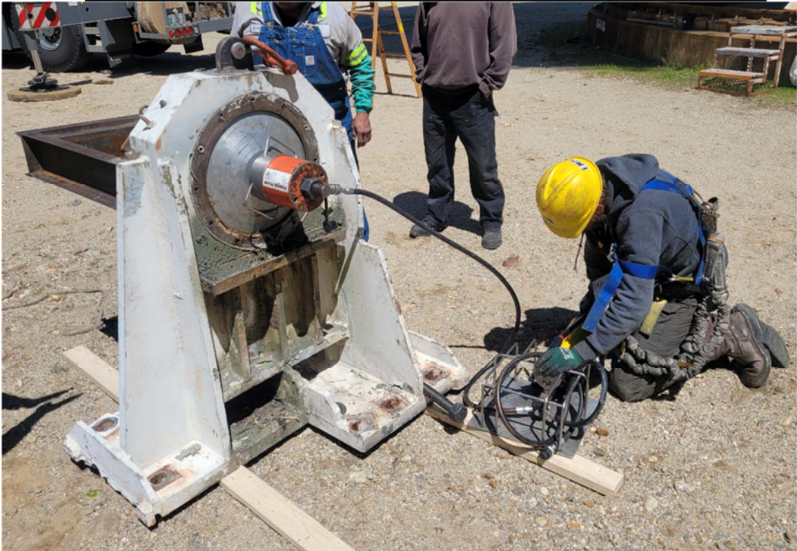
Figure 9: The bearing being pressed out of the block. The jack and pressure plate are used on the other side when pressing the new bearing into the block.
