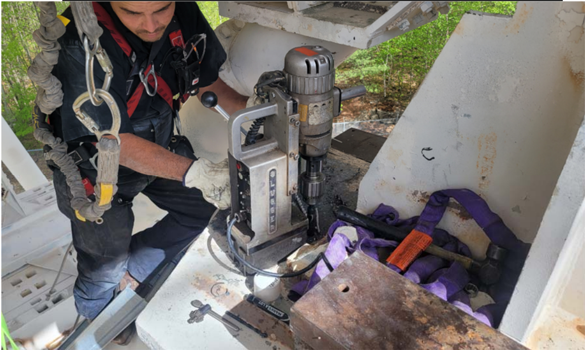
Figure 3: The encoder platform being drilled in preparation for installing the jack support beam.
