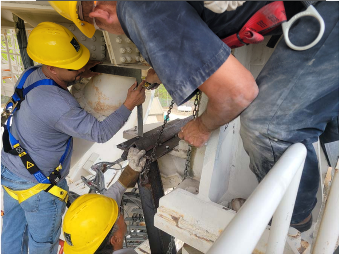
Figure 2: Scottin, Jason, and Patrick using the newly built template for marking the platform for drilling. Note that it is impossible to use it upside down.
