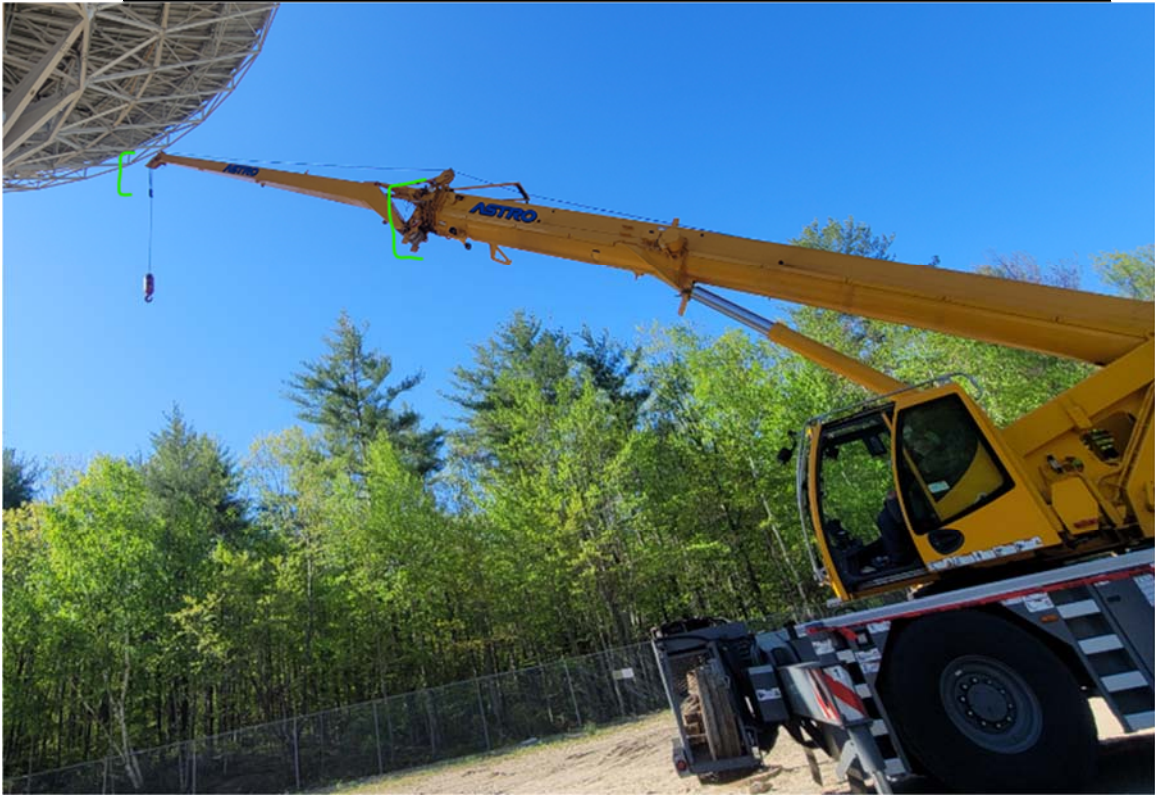
Figure 6: A comparison of the boom tip with or without the jib installed. With the jib installed, the height was much lower and allowed for extra maneuverability of the crane.
