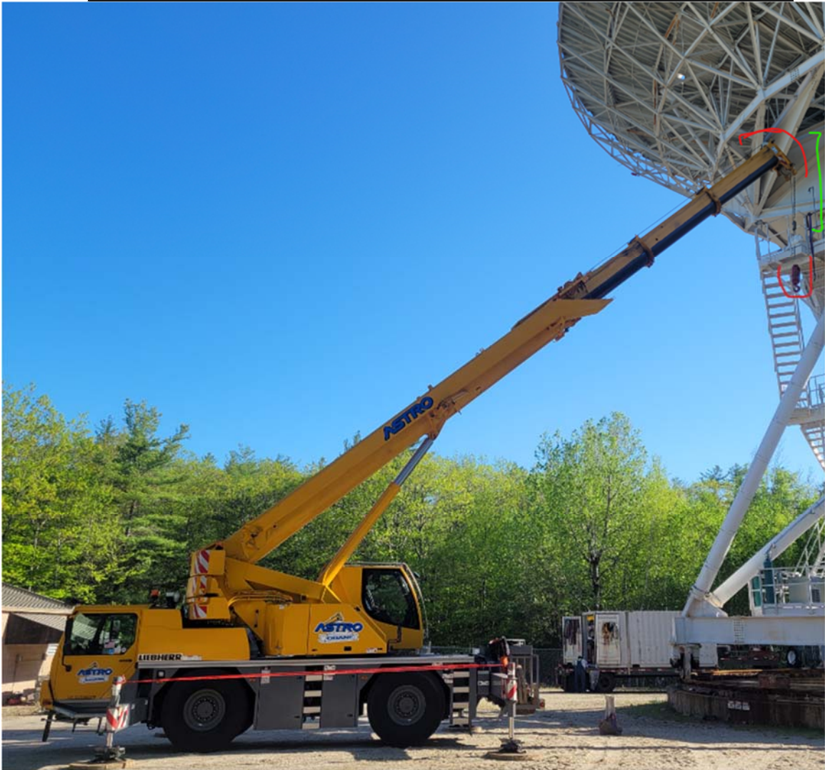
Figure 5: The crane without the jib installed. The hook and boom tip have been highlighted in red. The minimum height of the hook/boom tip are shown in green. This dimension was the greatest concern when renting an appropriately sized crane.
