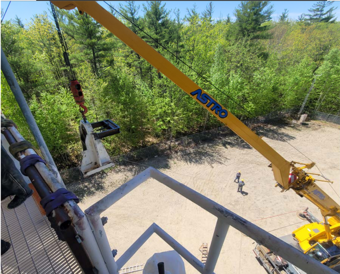
Figure 8: The pillow block being lowered from the platform. The crane operator showed 2700 lbs on the hook when the block was fully freed from the antenna.
