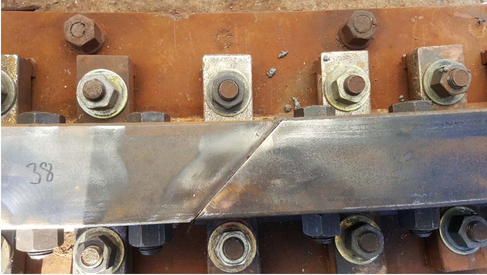
Figure 4.0.4: Bolt 38 Splice Gap.
