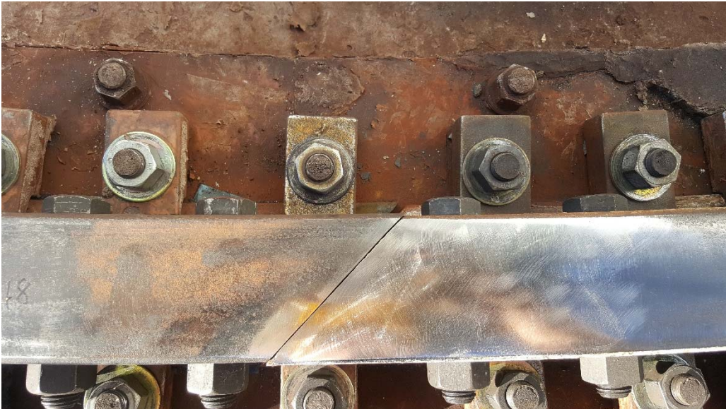
Figure 4.0.2: Bolt 17 Splice Gap.
