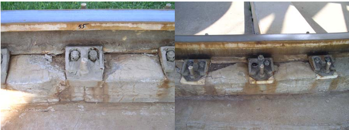
Grout has deteriorated from under the rail at bolt numbers 55 and 54. Rail clip bolts are broken at 34, 39 and 54.
