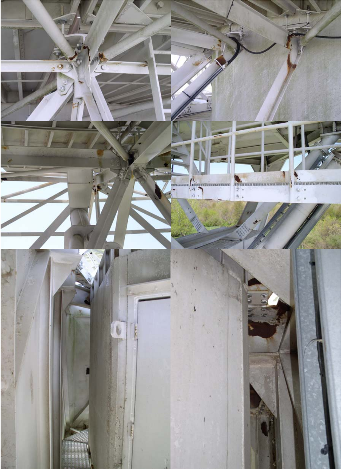
The Antenna could use a paint job. Paint is flaking off and surface rust is affecting most of the Antenna structure.
