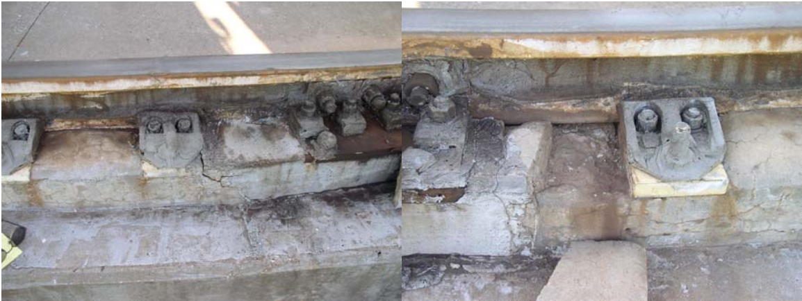
Grout is cracking and has fallen out at both ends of this rail splice. Bolt numbers 65 and 62.
