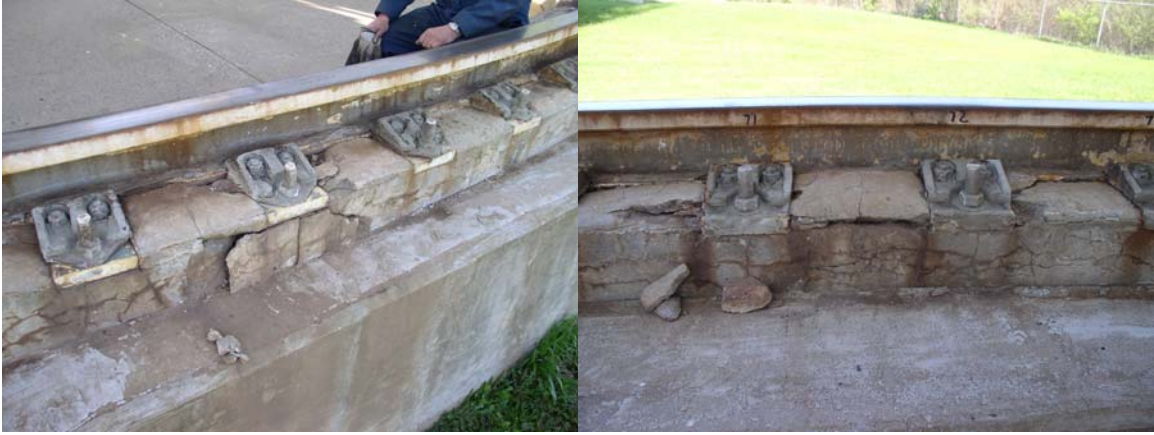
Grout is beginning to break up fall out from under the rail at bolt numbers 71 and 72.
