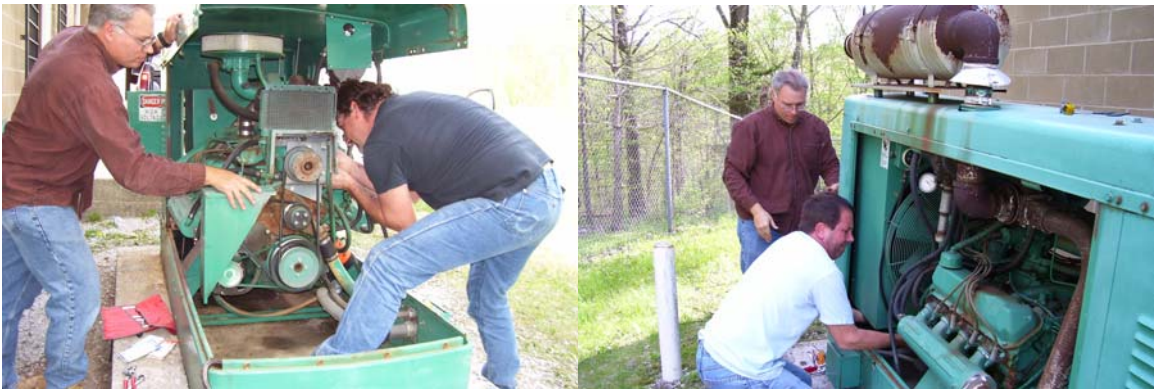
The Site Onan 75KW Generator radiator was repaired while the antenna was down for maintenance.
