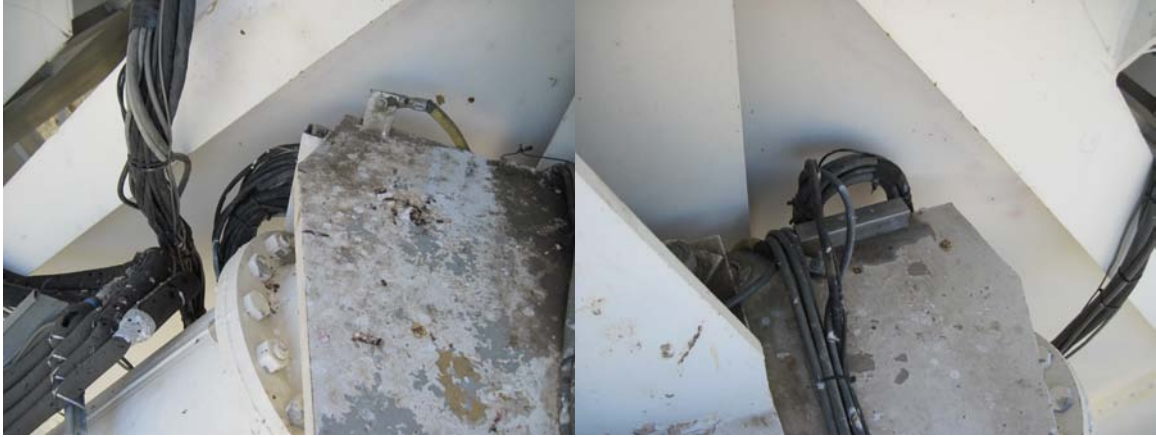
Both Elevation cable wraps are in good condition.
