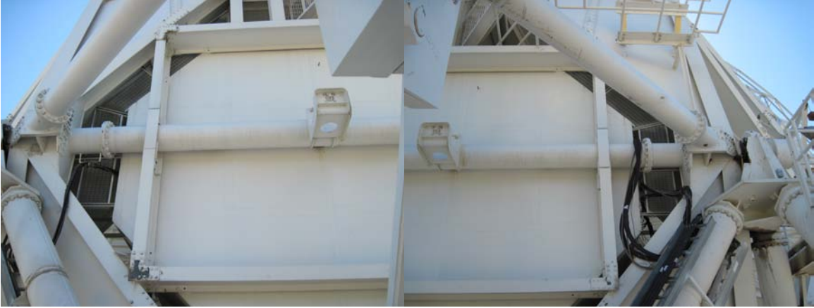
Elevation axle has no visible signs of cracks. Paint is in fair condition.
