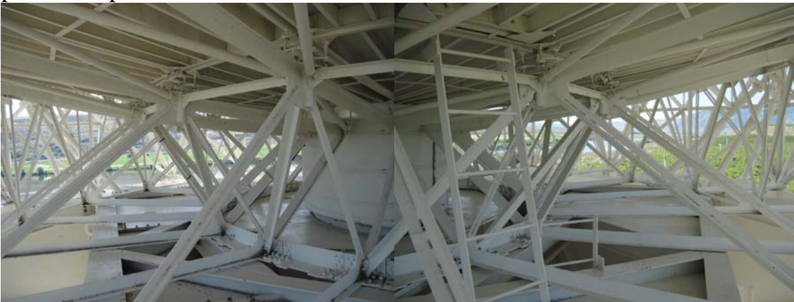
Antenna backup structure is in good condition. Paint is in fair condition.
