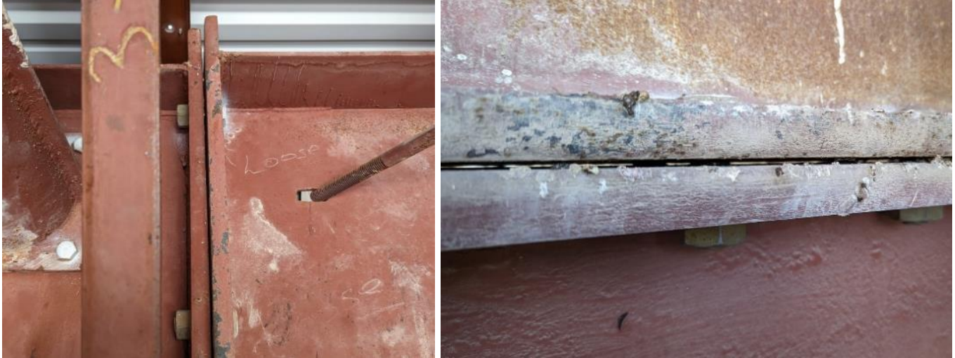
Figure 7: Left – Threads of bolt 5 are visible in gap (6e). Right – Bolts 1-4 & 24 were tight but had visible gaps. (13b)
