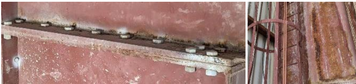
Figure 30: Typical corrosion found. Left – 6d. Right – 5b.
