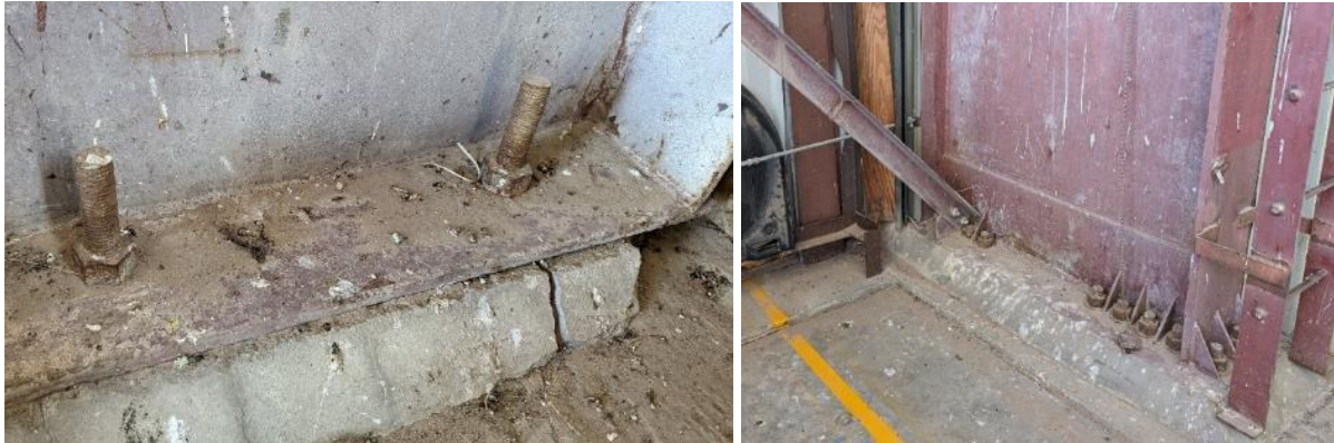
Figure 17: Left – CS2 foundation crack (8a). Right – Exposed section (4a).
