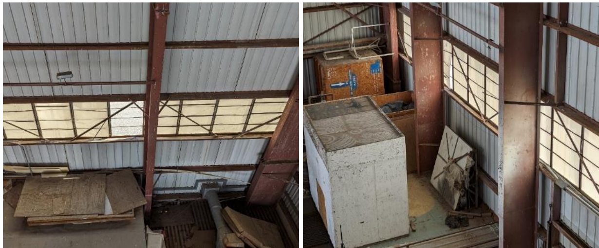
Figure 35: Left – Window panel missing (under 10b). Right – Window panel loose (under 7b).
