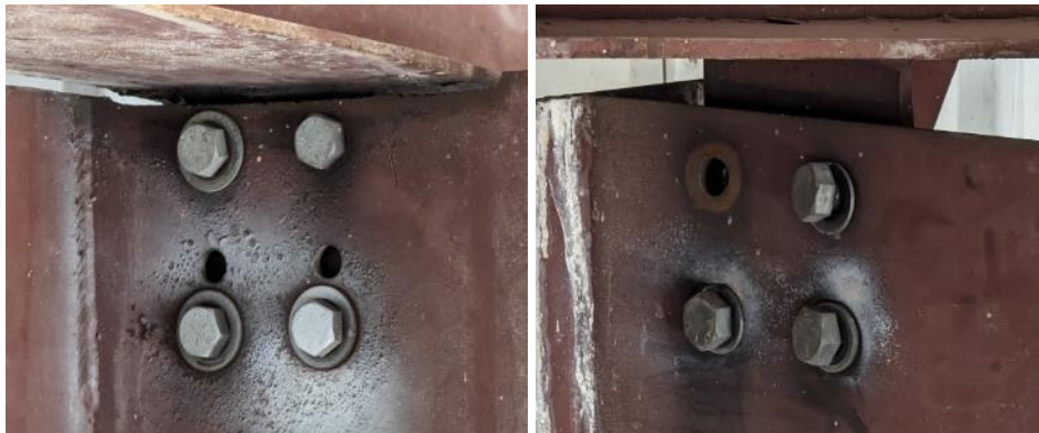
Figure 11: Visual comparison before tightening between 9d and 10d. Left – (9d). Right – (10d).
