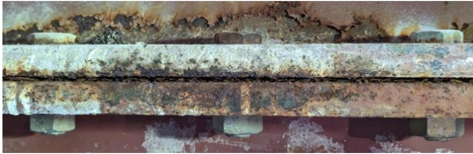
Figure 31: Corrosion found at 14d.
