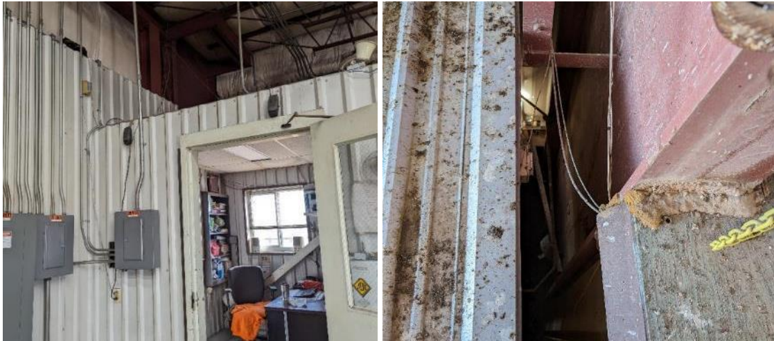
Figure 19: Section 5a unreachable. Left – Inside welding shop. Right – From welding shop roof.
