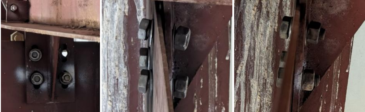
Figure 10: Left & Middle - Loose, missing, and misaligned bolts in connection (10d). Right – After initial tightening.
