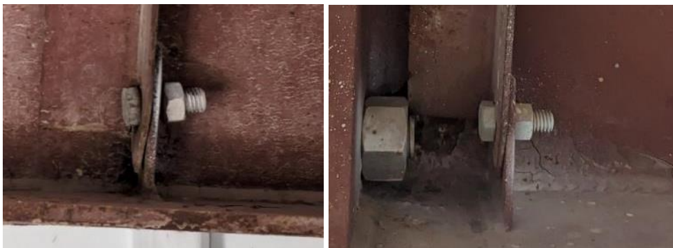
Figure 20: Typical flange brace bolting. Left – Flange brace 9 on south wall. Right – Near bolt 11 (2e).
