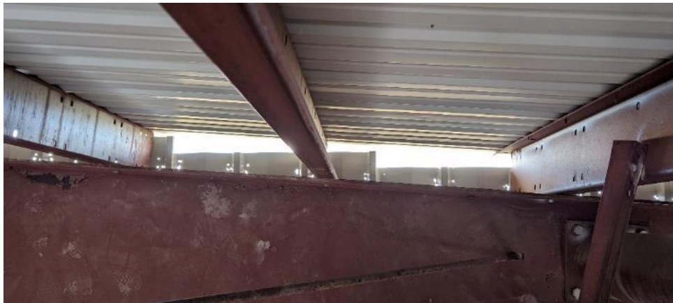
Figure 34: Large gap between roof and south wall (R-C5).
