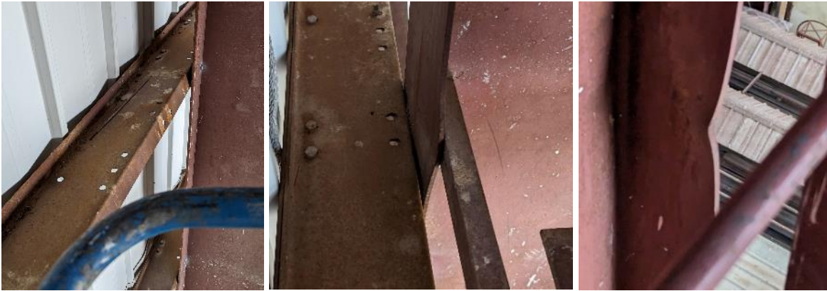
Figure 28: Left – Column is pushing into wall girt near 8c. Middle – Wall girt pushing into column at 2 nd ladder landing. Right – Slight buckling of column flange near 2 nd ladder landing.
