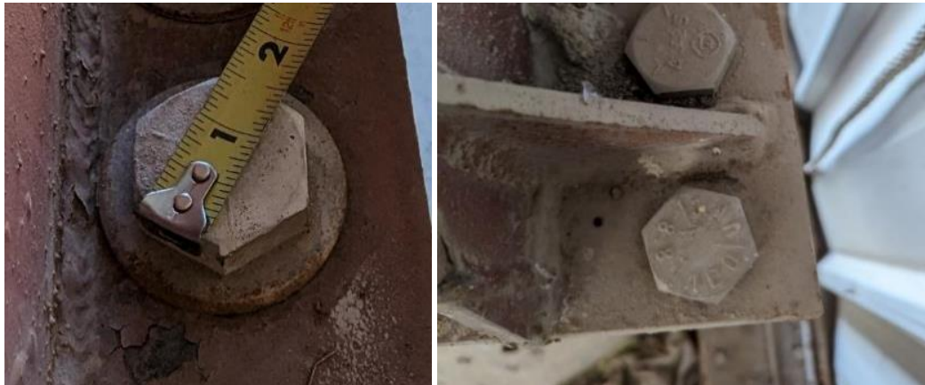
Figure 15: Left – Bolt 12 (14c) replaced with SAE grade 5 bolt. Right – Class 8.8 metric replacement of bolt 21 (5b). All f level bolting sections appeared to be in good condition, with no signs of looseness or damage.
