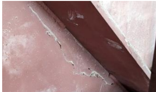
Figure 29: Typical surface cracks of paint (5d).
