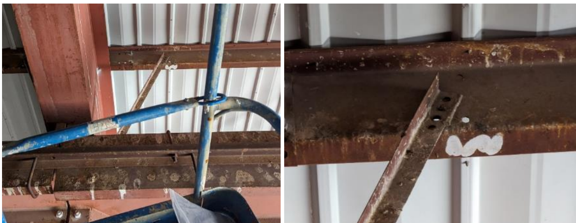
Figure 25: Missing 1/2" bolt for flange brace under 15d.
