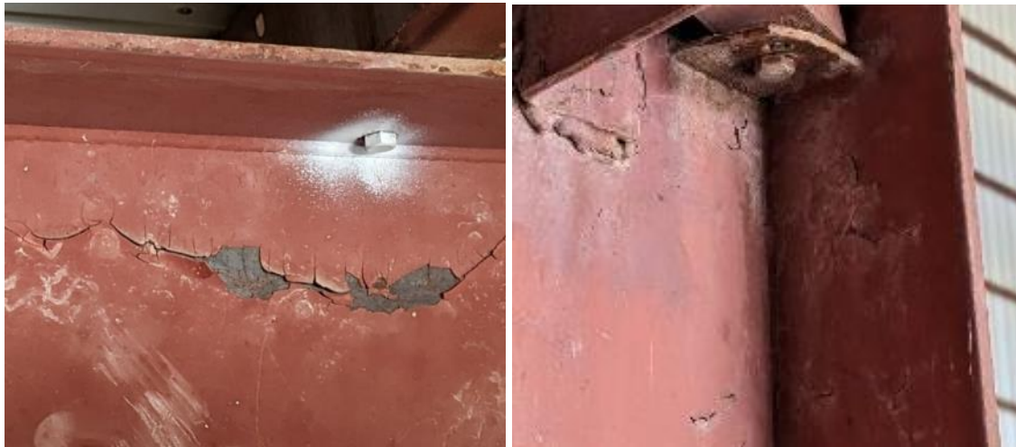
Figure 27: Left – Between 6d and 6e. Right – Near horizontal flange brace under 5c.
