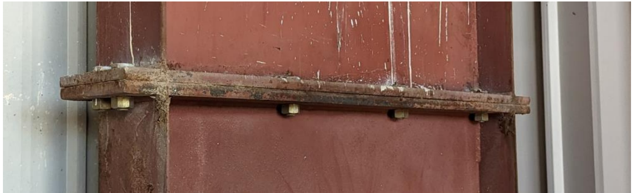
Figure 2: Image of bolts with zinc coating (11c)
