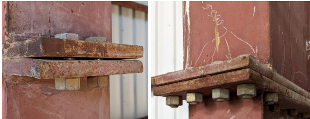
Figure 8: Left – Bolts 6 & 7 rotated about 15 degrees (4c). Right – (7c)
