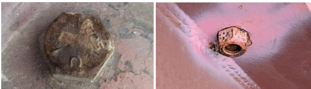
Figure 9: Bolt 18 (1b) found to be heavily corroded and short.
