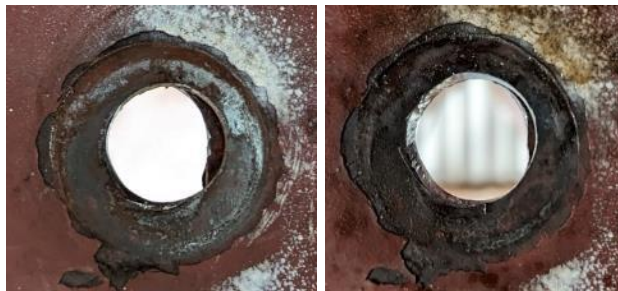
Figure 14: Visual clearance of bolt 4 (7d) Left– Before die grinding. Right – After die grinding.
