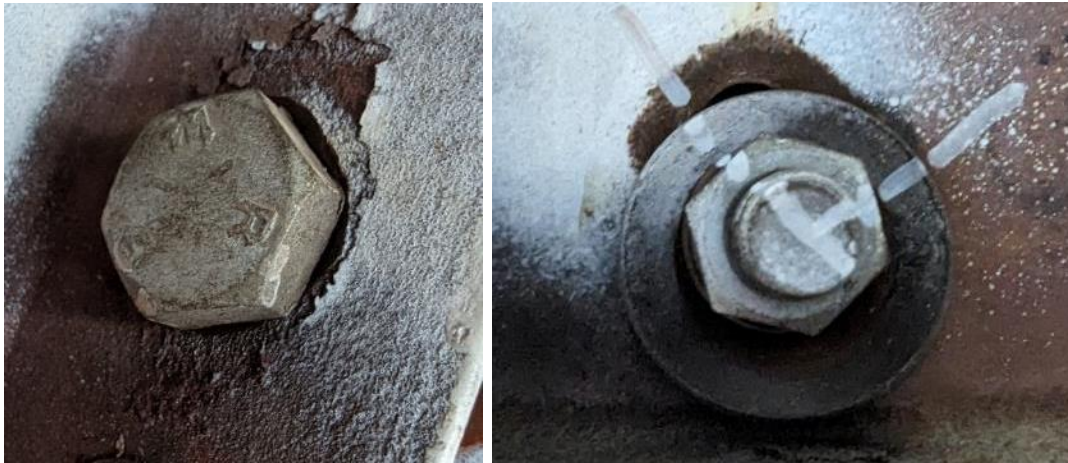
Figure 21: Top bolt in flange brace 10. Left – View of head. Right – View of nut double match marked.
