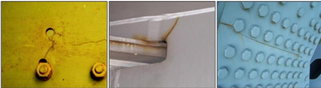
Figure A10: Corrosion and cracking examples.
