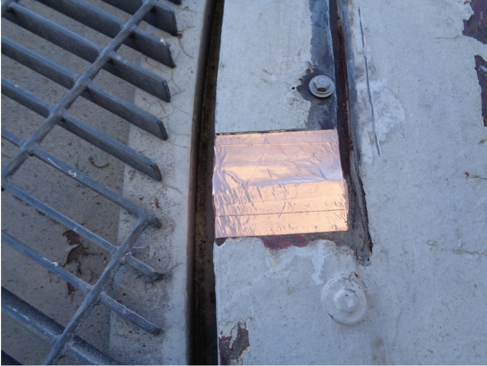
New copper tape over joint section. Ready to apply new caulk and paint:
