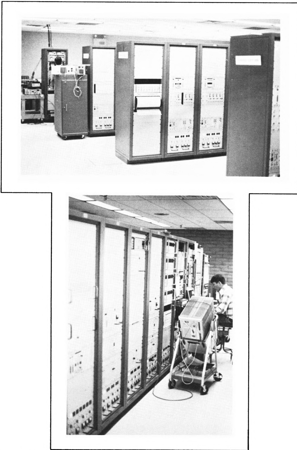
Figure 3-3. Two photographs of the central electronics room. The top picture shows the D-racks for each arm and the bottom photograph shows the row of racks containing the Master LO system, the Monitor and Control Interface, and the phased array output racks.
