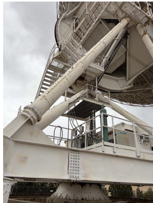
Figure 29: Quadrapod Support Insulation
