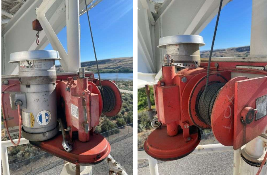
Figure 23: Jib Crane on the Elevation Encoder Deck
