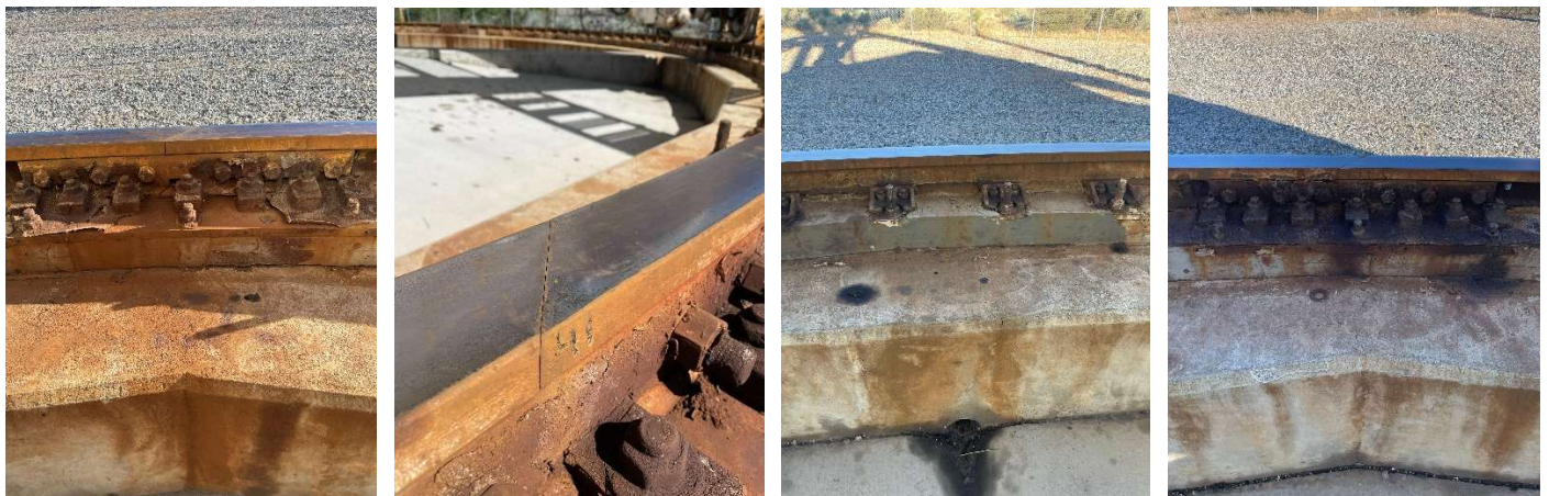
Figure 3: Rail System Condition (Bolt #1, #41, #92 and #101, respectively)
