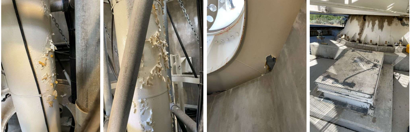
Figure 12: Pintle Bearing Room Access Hatch, Cable Wrap and Port Hole
