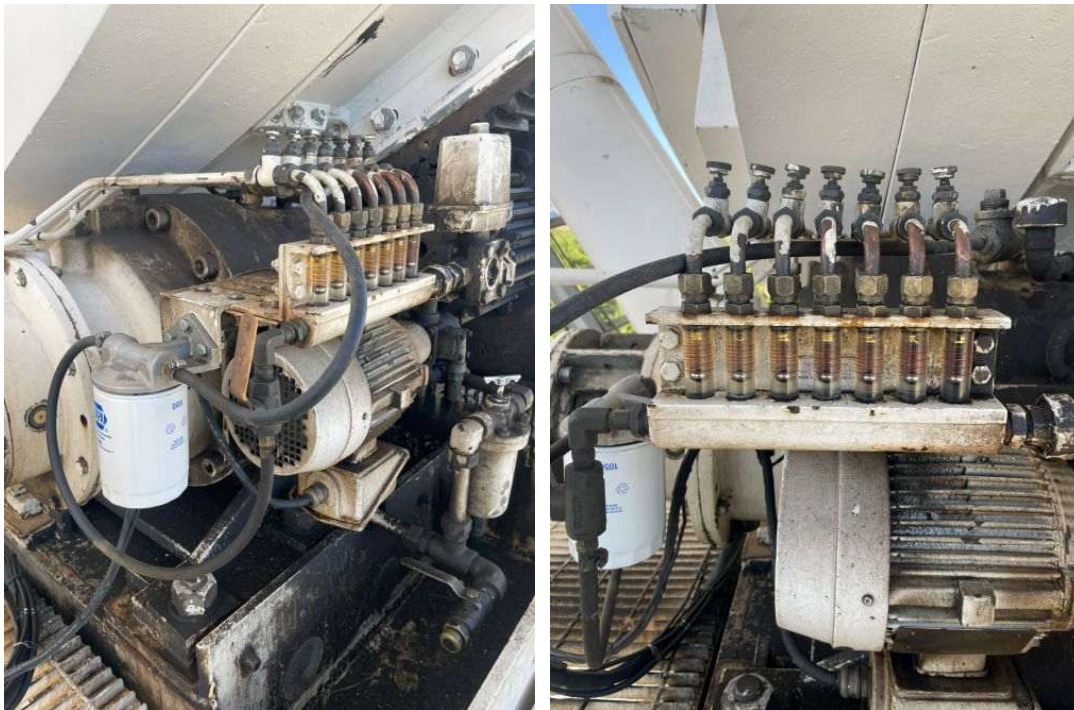
Figure 19: Elevation Drive EL1 Bypass Hose Lines and Filter Lines
