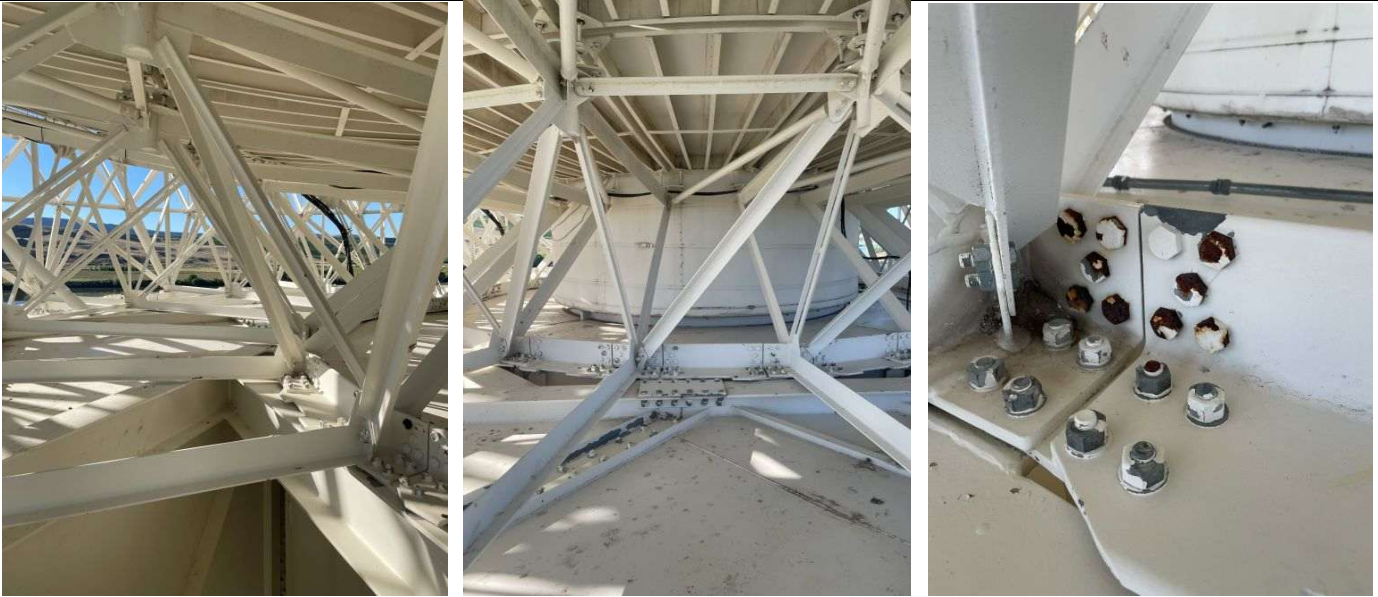
Figure 26: Main Dish Backup Structure Central Frame and Fasteners
