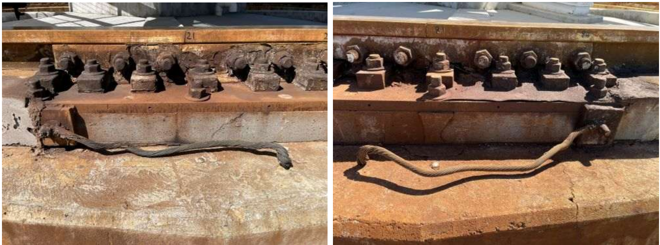
Figure 9: Rail Ground and Grounding Wires
