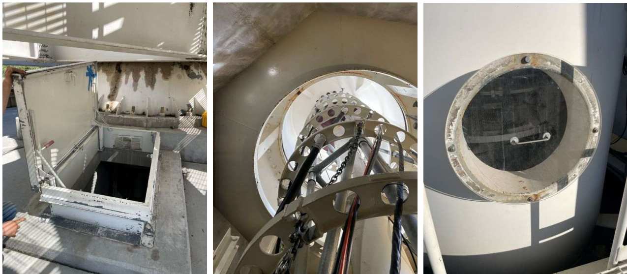
Figure 11: Pintle Bearing Room Access Hatch, Cable Wrap and Port Hole
