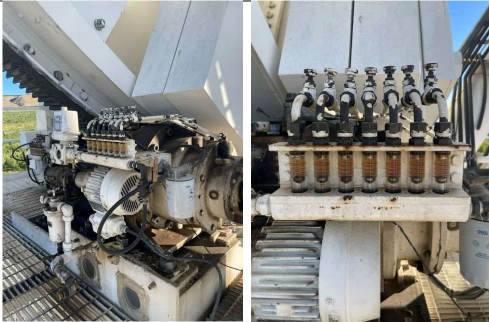
Figure 20: Elevation Drive EL2 Bypass Hose Lines and Filter Lines
