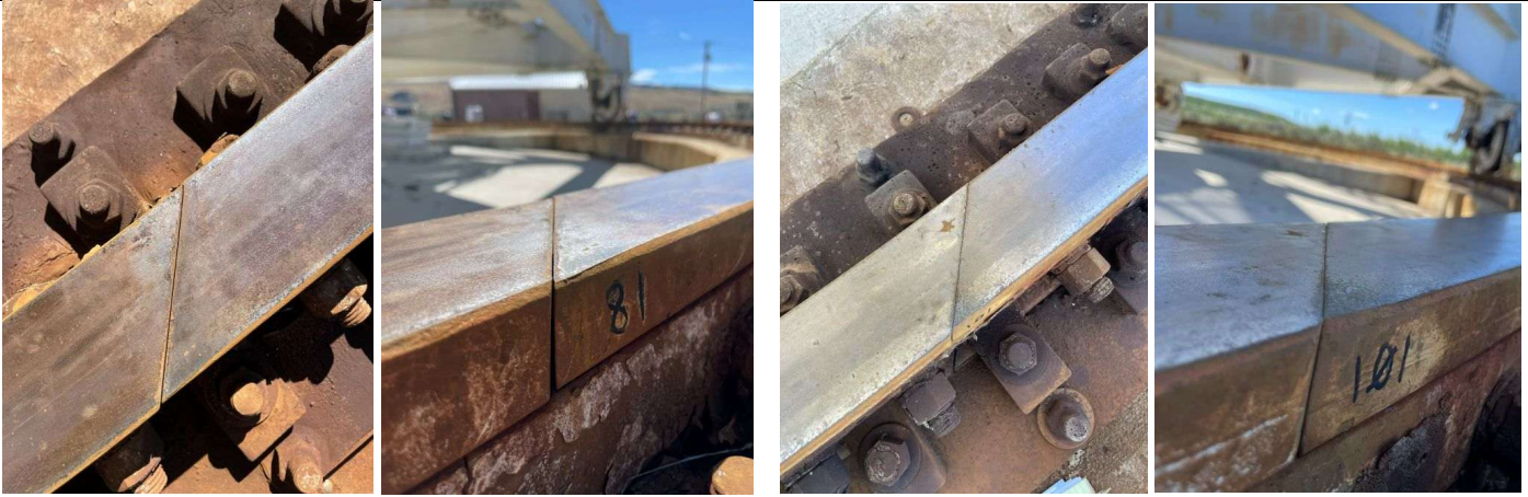
Figure 6: Rail Gaps (Bolt #81 and #101, respectively)
