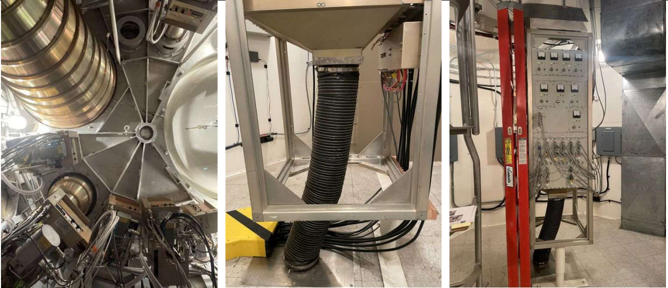
Figure 24: Views of Vertex Room
