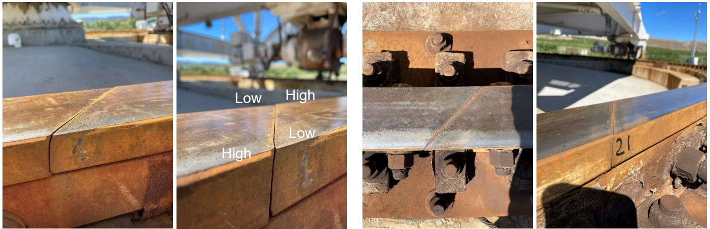
Figure 4: Rail Gaps (Bolt #1 and #21, respectively)
