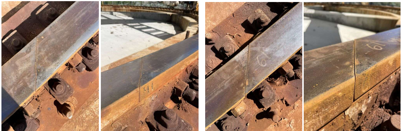
Figure 5: Rail Gaps (Bolt #41 and #61, respectively)
