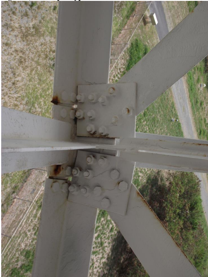
Figure 6., Minor corrosion due to paint thinning on edges.
