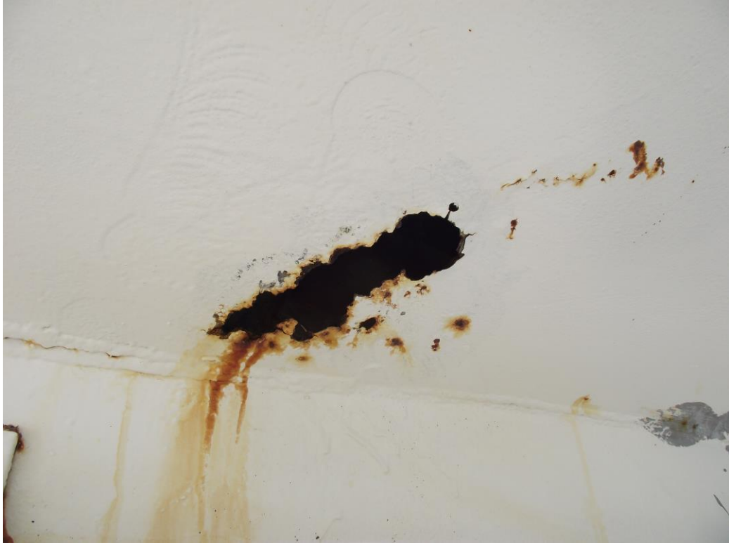
Figure 9, Corroded drain hole that will need repair.
