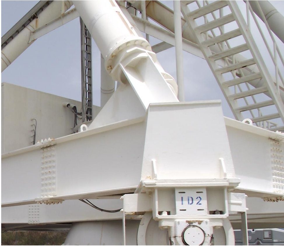
Figure 17, Support structure corrosion is minimal.
