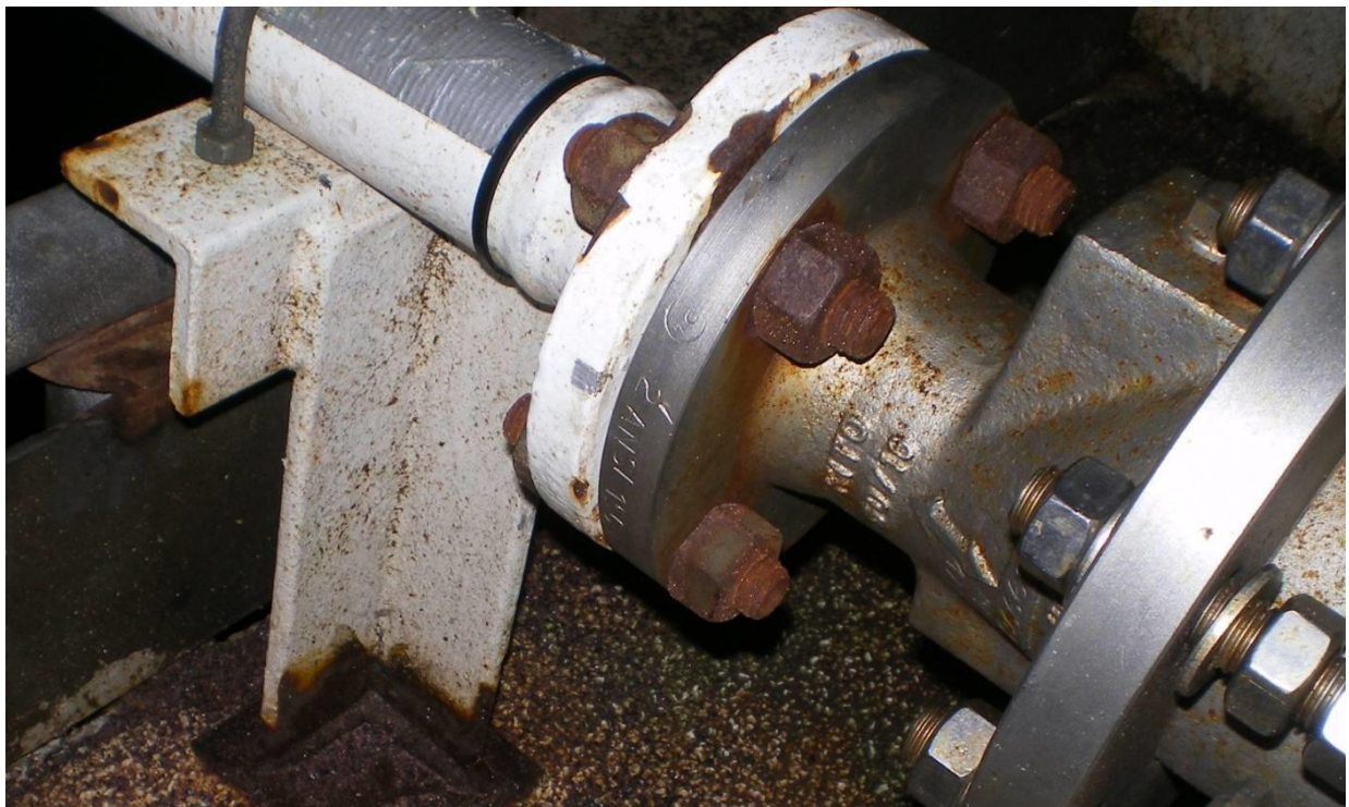
Figure 1: corroding low-alloy bolts in contact with high-alloy components
