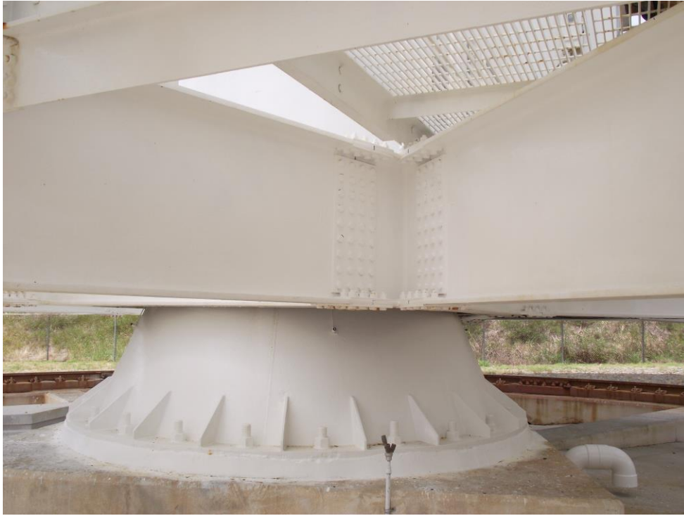
Figure 19, Pintle bearing housing corrosion.
