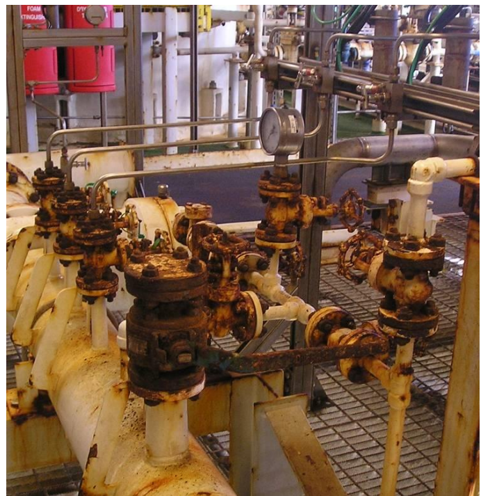
Figure 8: rusting flanges on a North Sea platform
