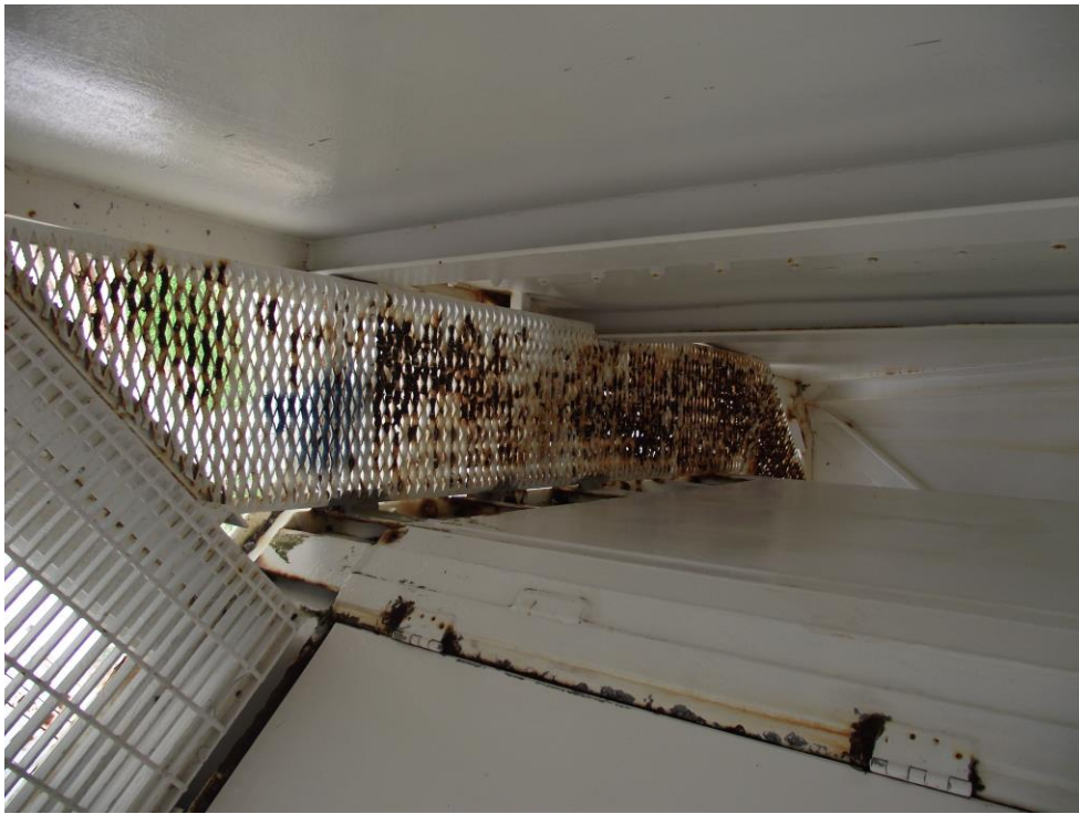
Figure 14, Lightweight walkway grating around vertex room is failing and will need to be replaced.
