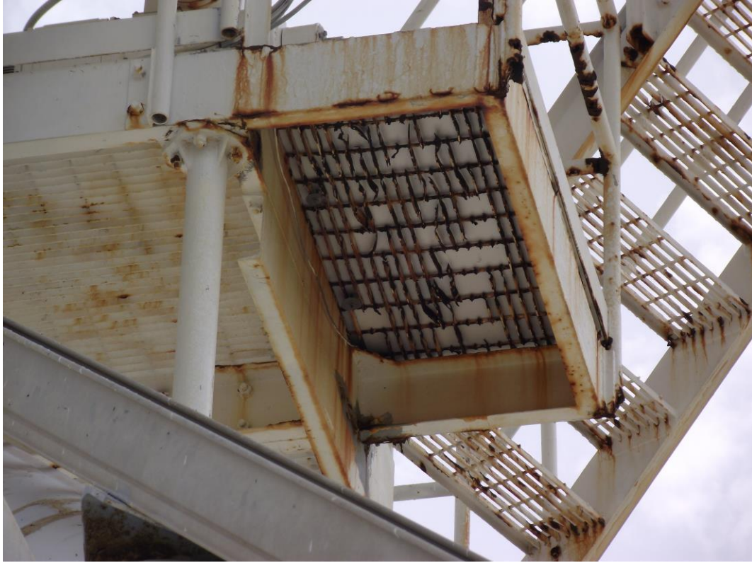
Figure 13. Example of failed bar grating.
