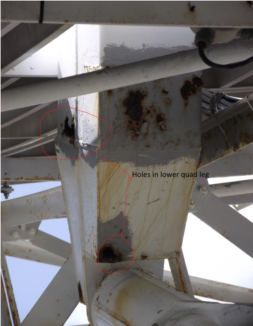
Figure 2, Quad leg corrosion below dish
