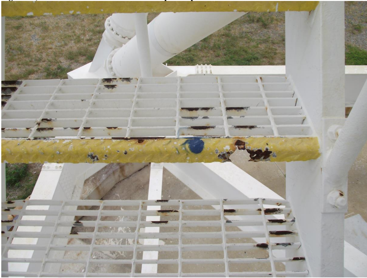
Figure 16. Stair nose that requires replacement.
