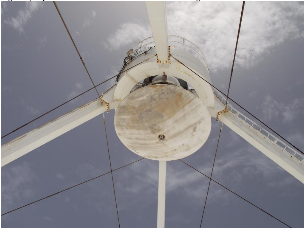
Figure 2, Rust staining on bolted connections at apex. Subreflector paint condition
