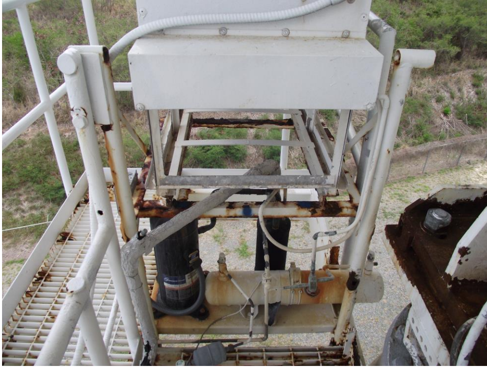
Figure 21, HVAC condenser platform.
