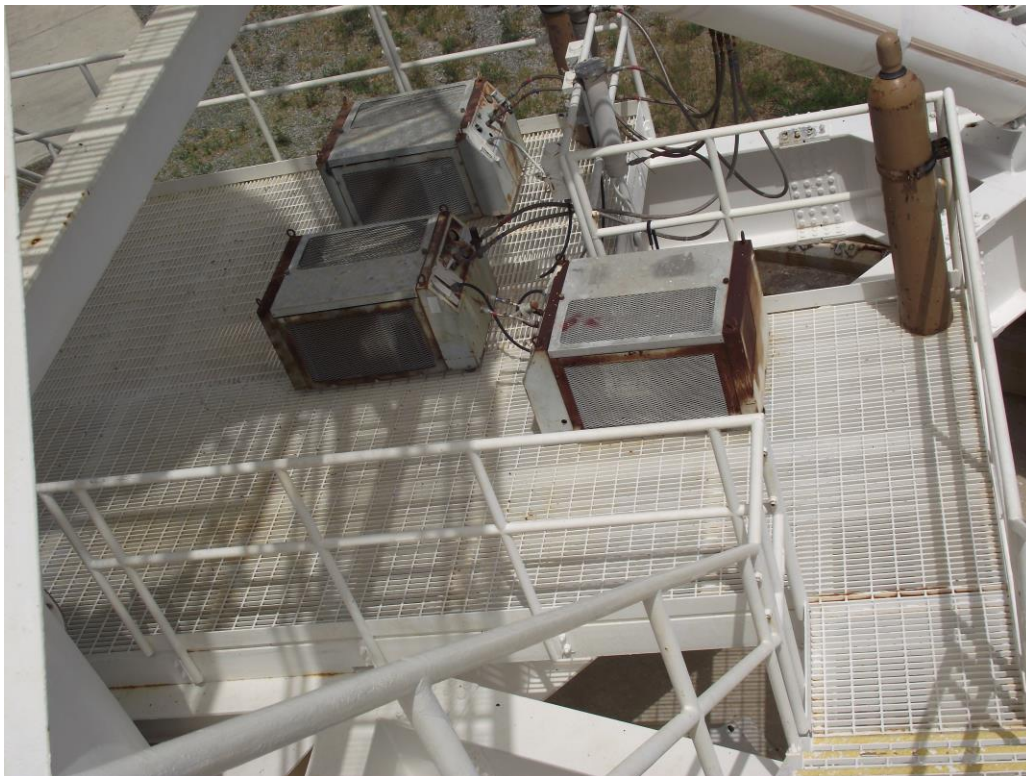
Figure 12. Typical paint condition on bar grating and hand rails.
