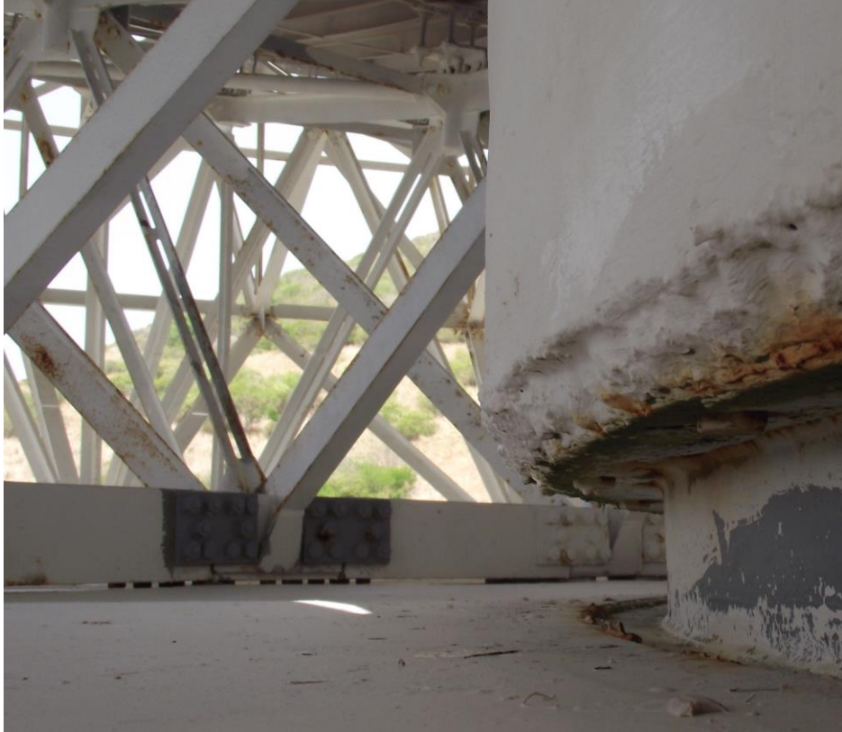
Figure 7, Vertex room bolt corrosion.
