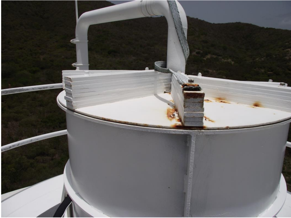
Figure 1, Superficial corrosion at FRM barrel counterweights.
