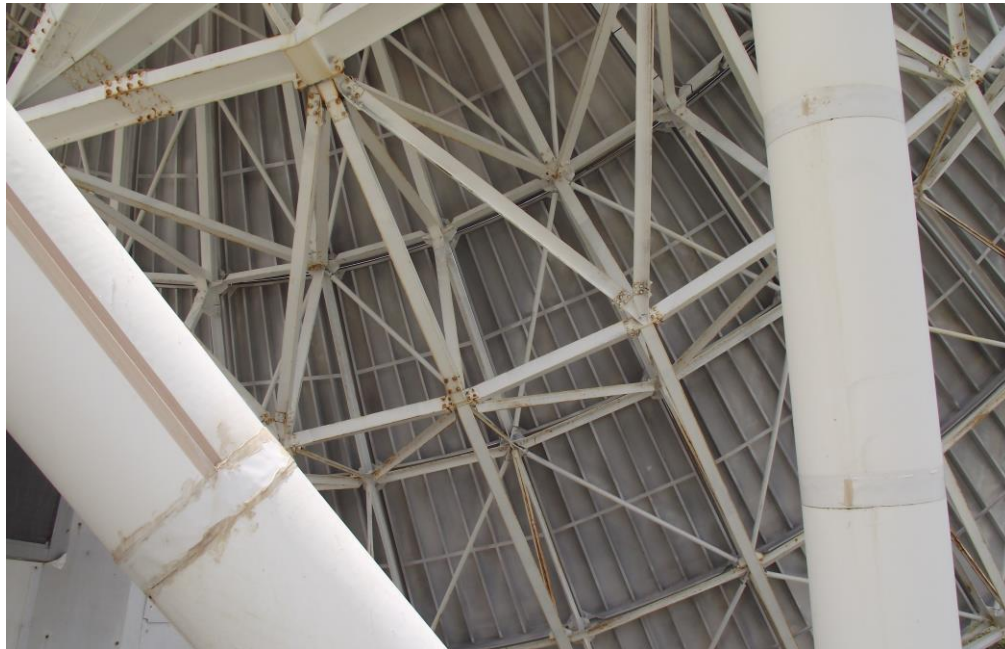
Figure 4, Extent of rust stained bolts.
