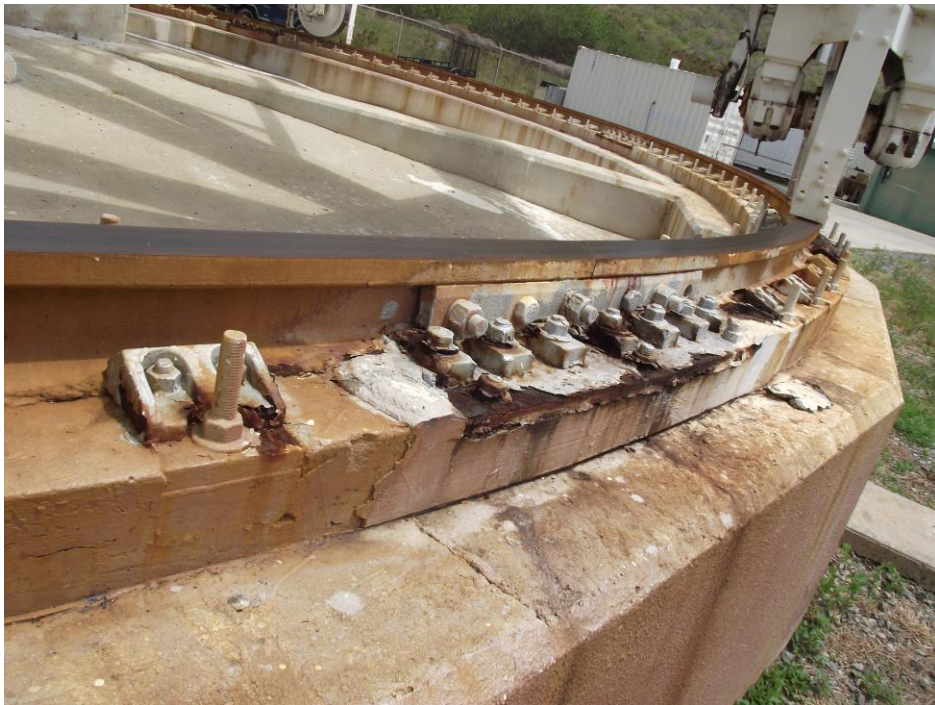
Figure 18, Corrosion on rail, rail clips and splice plates.
