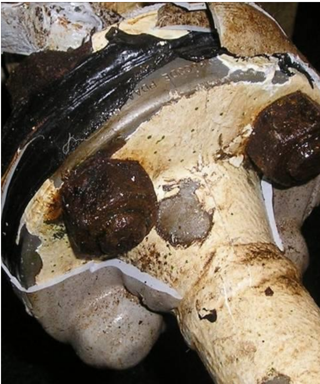
Figure 11: after 2 years oil-soaked substrate shows no further corrosion 7 years with CIST
