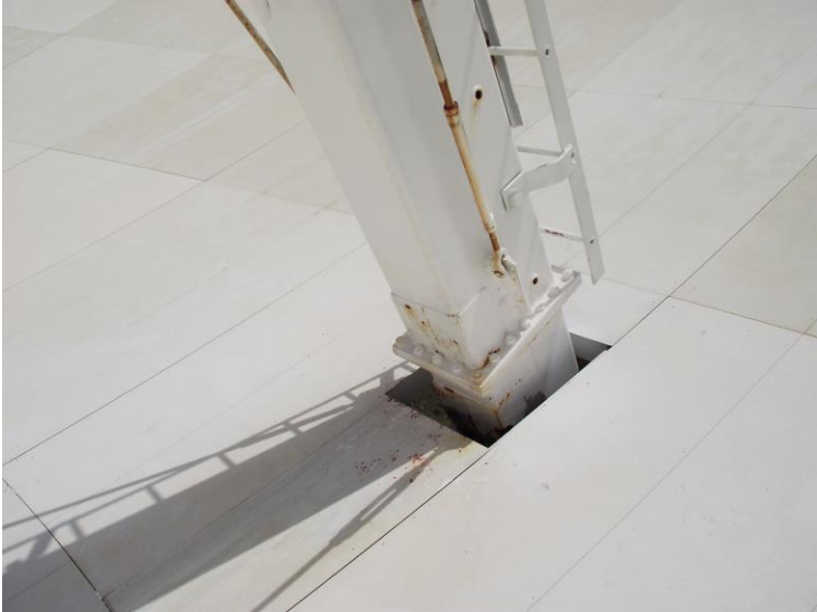
Figure 1, Quad leg corrosion above the dish.
