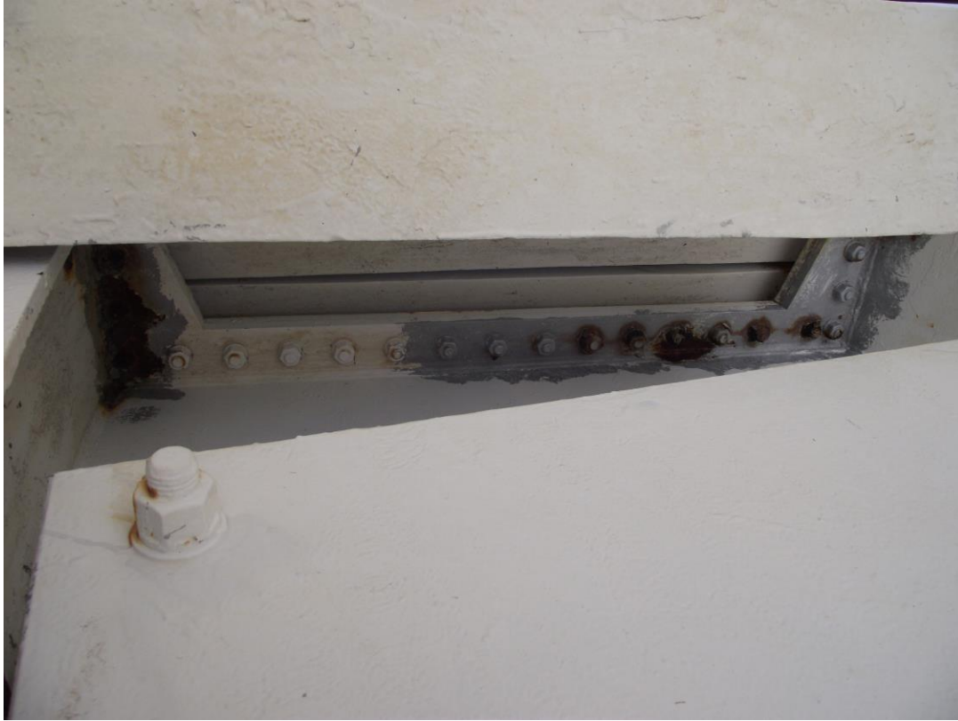
Figure 11, Counterweight bolts. Corroded section on left is where the site techs needle scaled the corrosion and have not yet repainted.
