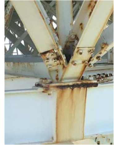
Figure 8: Structural Connection that Ponds Water
