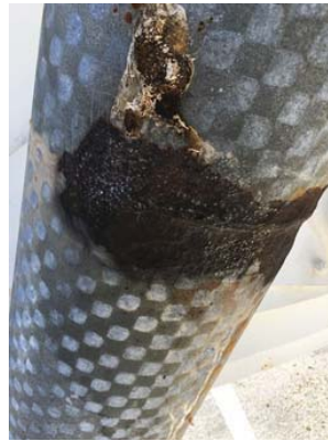
Figure 4: Typical Corrosion at Bracket Connection
