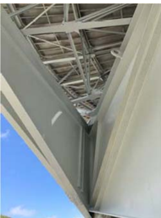
Figure 10: Antenna Support Structure with Top Coat
