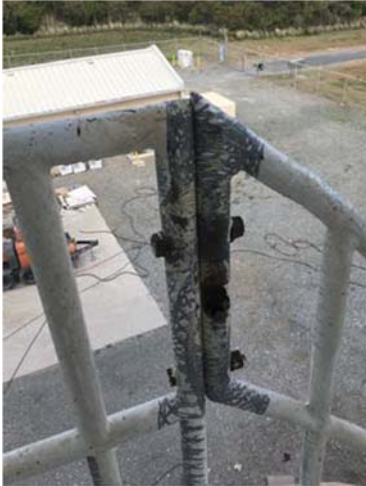
Figure 9: Typical Hand Rail Corrosion
