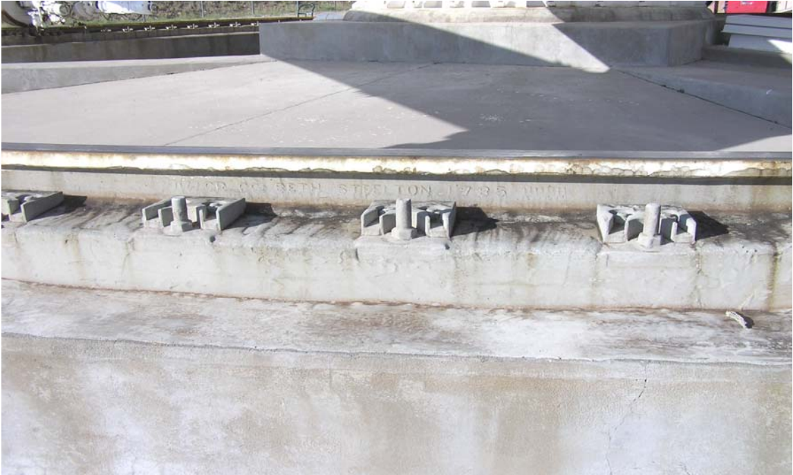
Vulchem is deteriorating off rail clips and will have to be removed.
