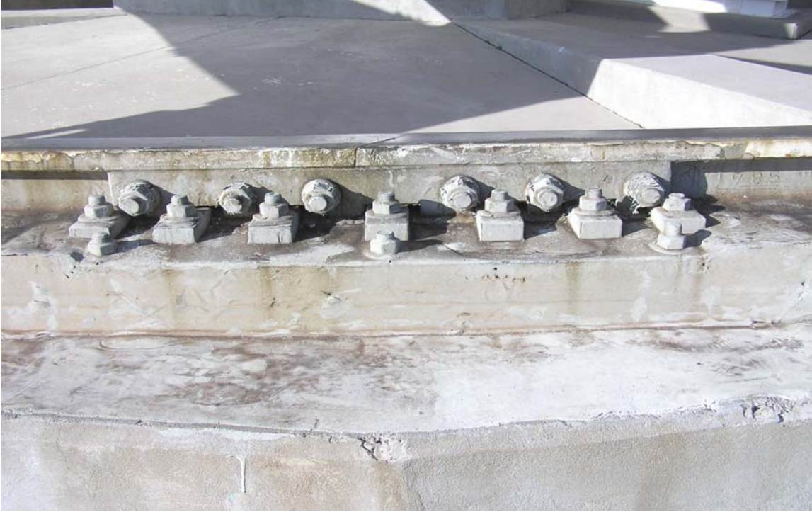
Vulchem is beginning to deteriorate from this rail splice and all others.
