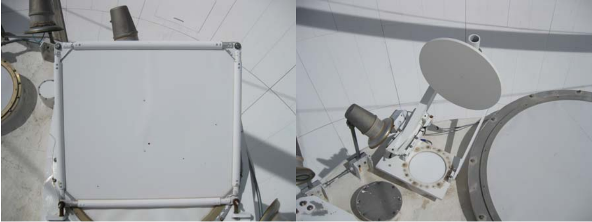
The Dichroic reflector is in good condition. The Ellipsoid reflector is in good condition. Ellipsoid actuator operates correctly.
