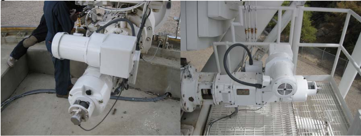
Azimuth #1 blower motor and spider coupling was replaced. Elevation # 2 motor was replaced.
