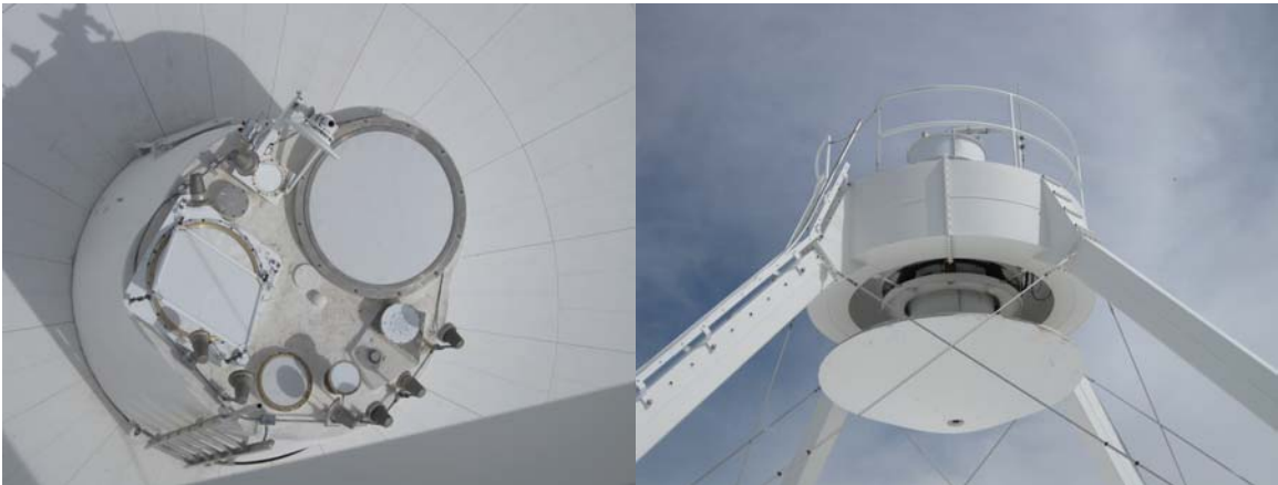
The feed heaters and FE windows are in good condition. Apex paint is in good condition.
