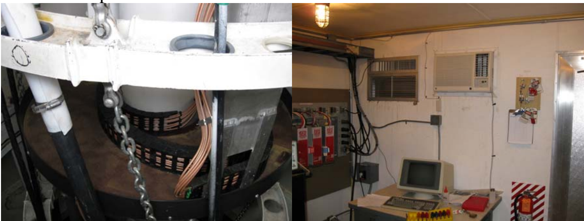
The new IF cable wrap is in good condition. The ped room Marv Air, air condition compressor failed. It was removed and brought back to the VLA for repair.
