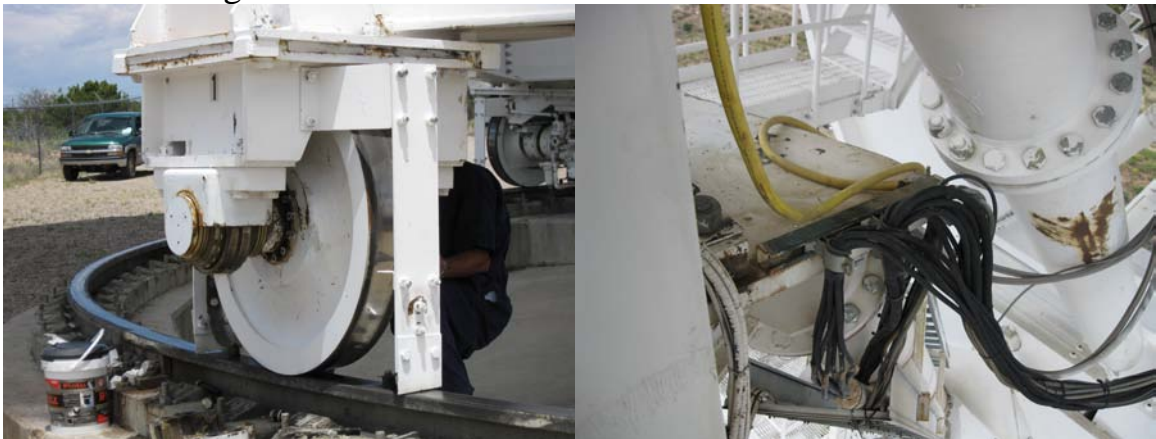
AZ and EL bearings were inspected. Both Elevation cable wraps are in good condition.
