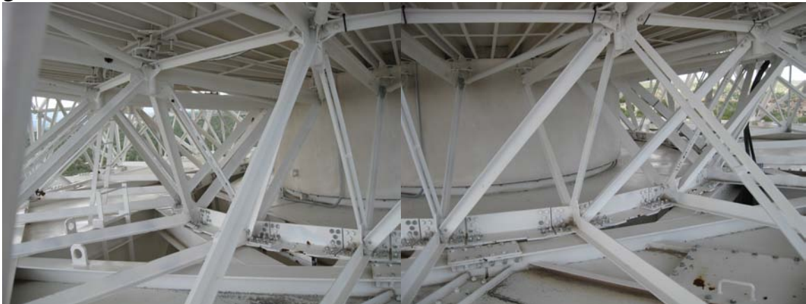
Antenna backup structure is in good condition. Paint is in good condition.
