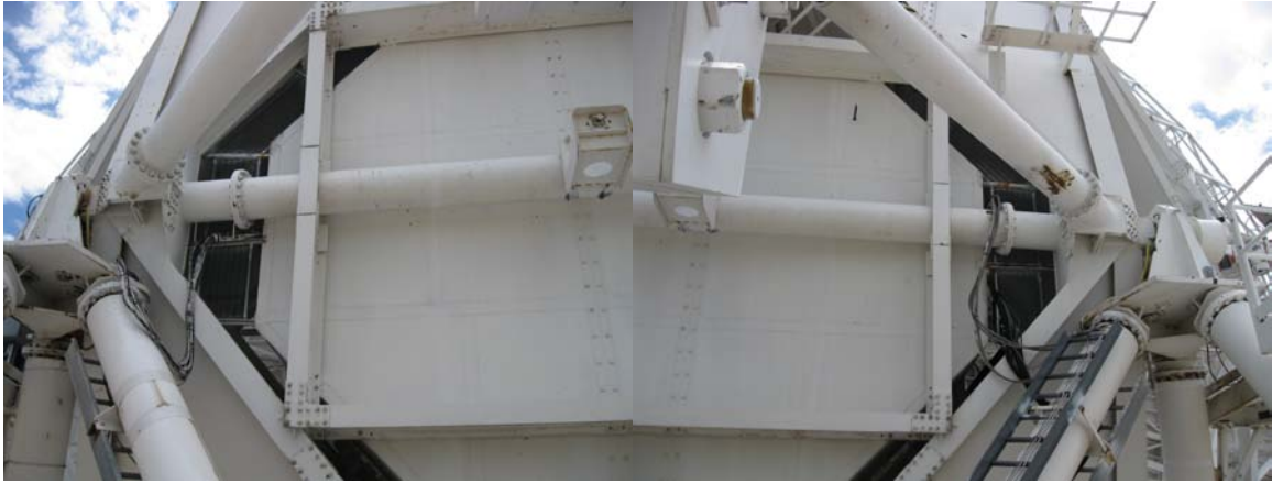
Elevation axle has no visible signs of cracks. Paint is in good condition.
