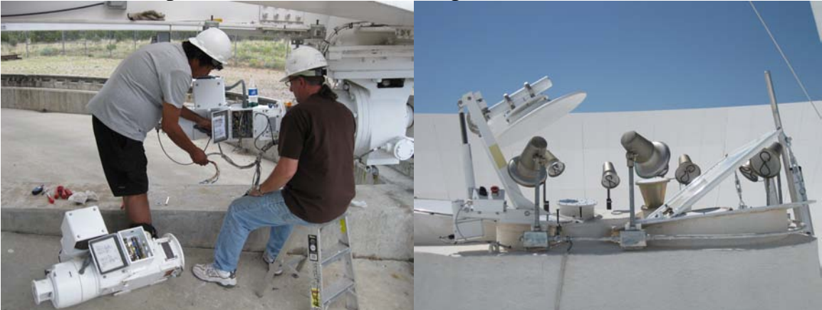
Azimuth #1 motor was replaced. The Ellipsoid reflector is in good condition. The ellipsoid actuator operates correctly.
